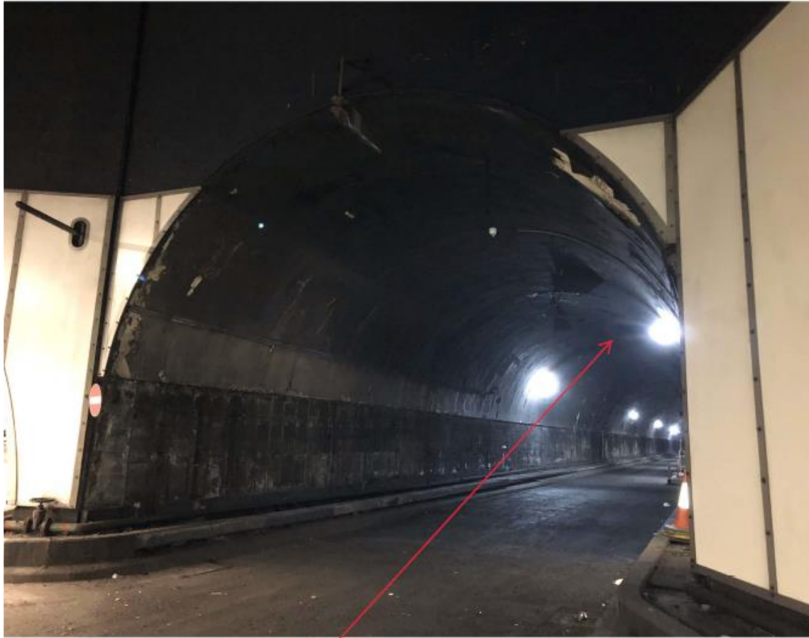
jet fan position approximately 25m inside Rendel Street Branch Tunnel
